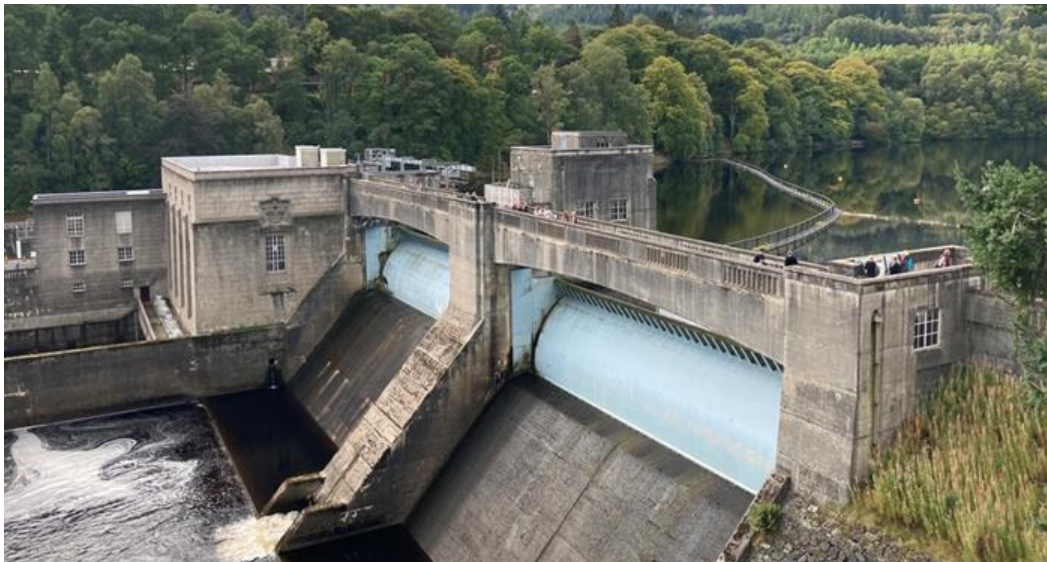
Example of a RCC Dam - Photo of Pitlochry Dam with Spillway (taken 2022)
