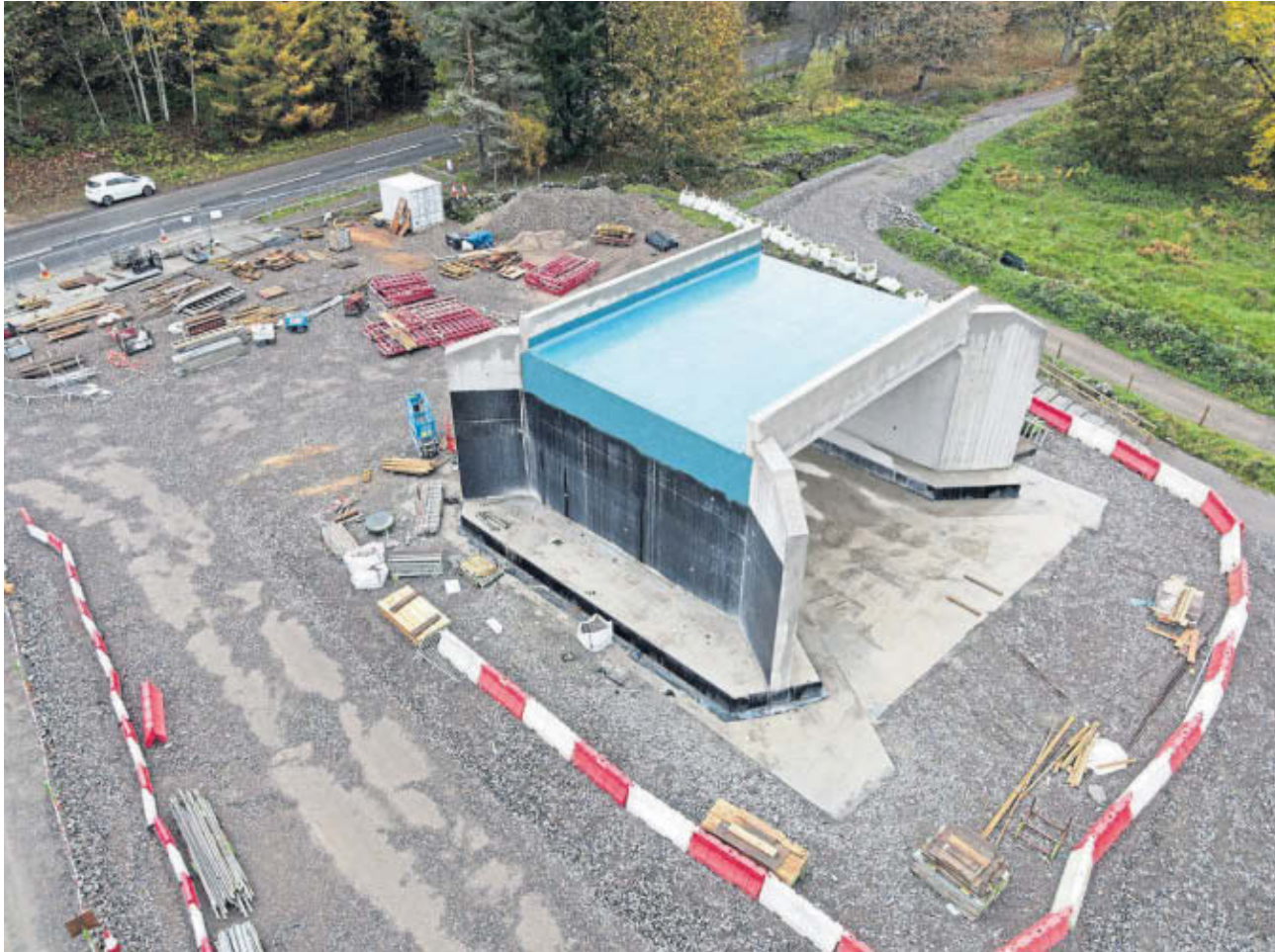
PREFAB BRIDGE: The replacement bridge to be installed at Lynebeg has already been constructed nearby.
